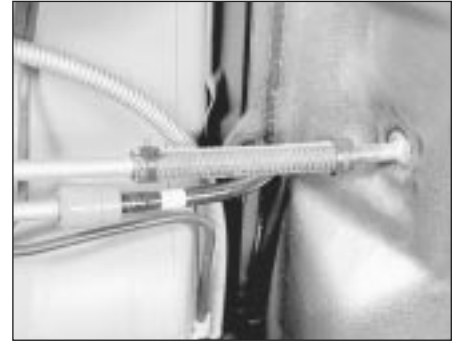
6.3 Fuel tank flexible hose connections at front of tank
